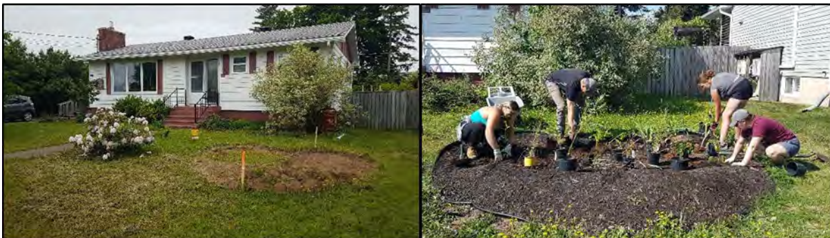
Before (left) and during (right) construction of the rain garden on Rue Louisiane
