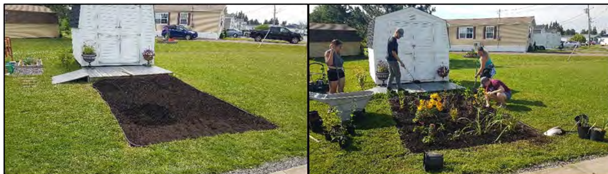
Before (left) and during (right) construction of the rain garden on Rue Grand Pré.
