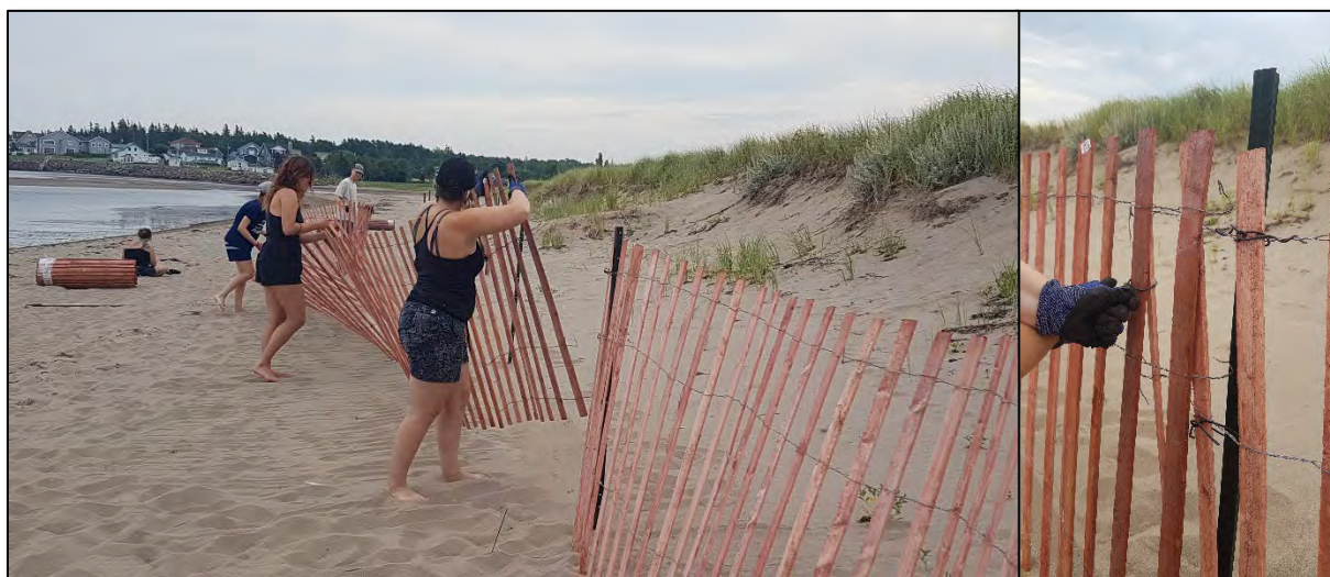
Figure 37: SBWA summer students installing dune fencing (left) and secured to t-post (right)
