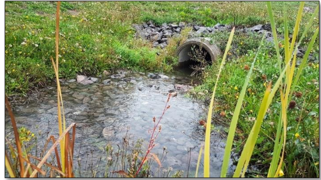
Figure 5: Bioretention System – Water Inlet
