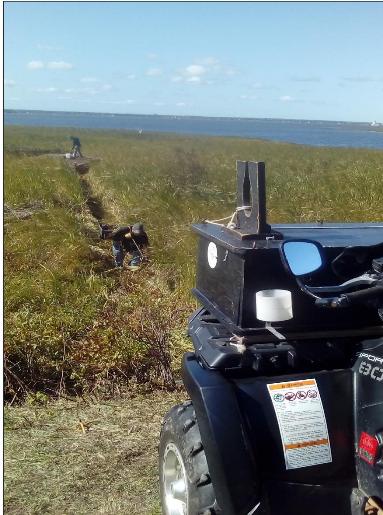
Figure 10: Path we used to carry, drag, and winch demolished sections of old nesting platform
