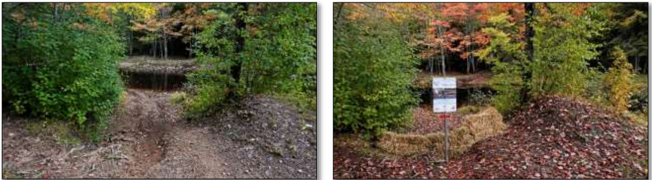
Figure 12: Before and after photos of ATV access blockage and sediment control (hay-bale check dam)
