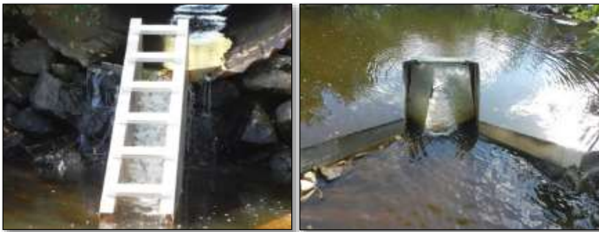
Figure 18: Up-close view and overhead view of the fish ladder with water deflectors
