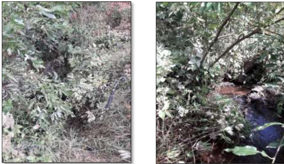
Figure 26: Before and after photos of the shrub thinning upstream of the culvert
