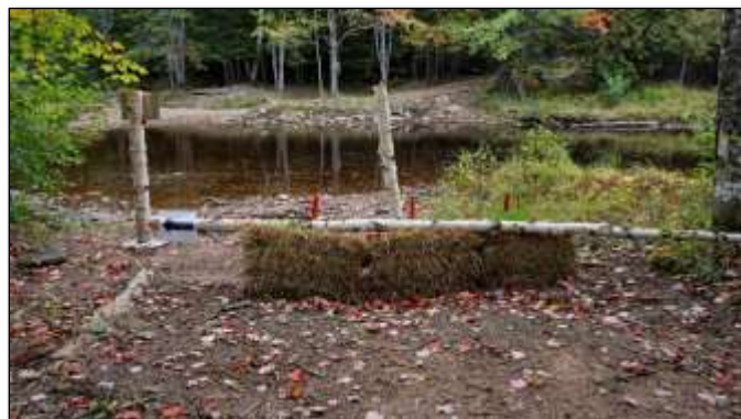
Figure 23: ATV access blockage and sediment control (hay-bale check dam)
