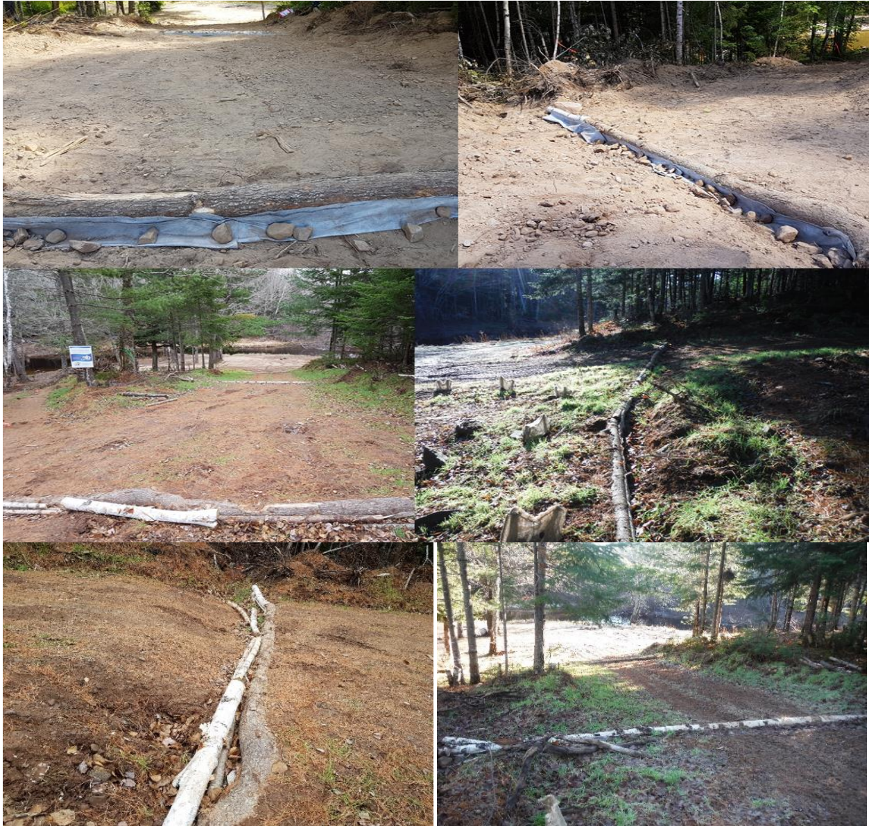
Figure 20: Photos of the sediment deflector logs at the Scoudouc River restoration site, 2017
